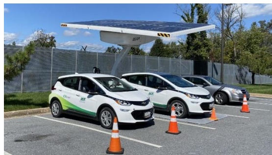
Fig 3.1 Renewable Charging Stations
