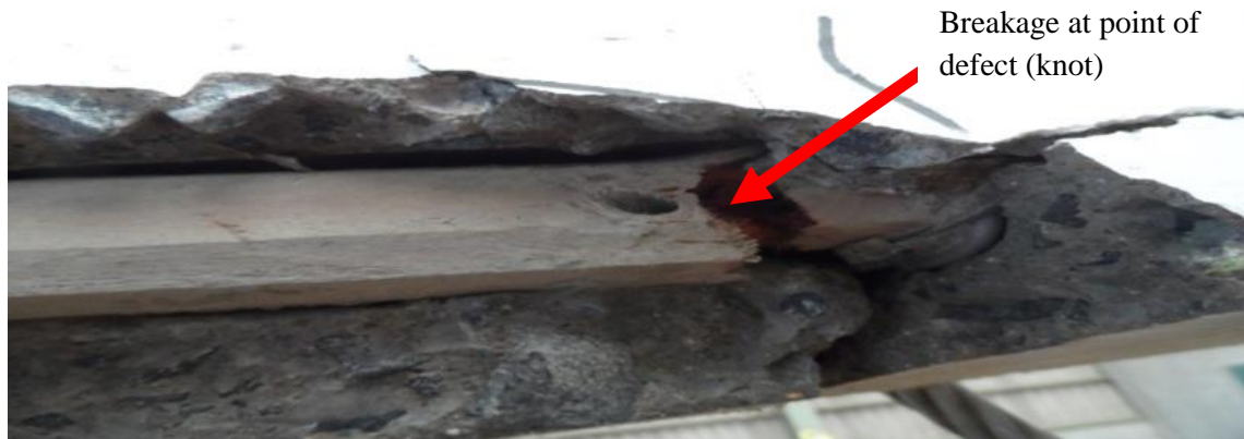
Figure 8: Crack of Mangrove Pole inside the Beam
